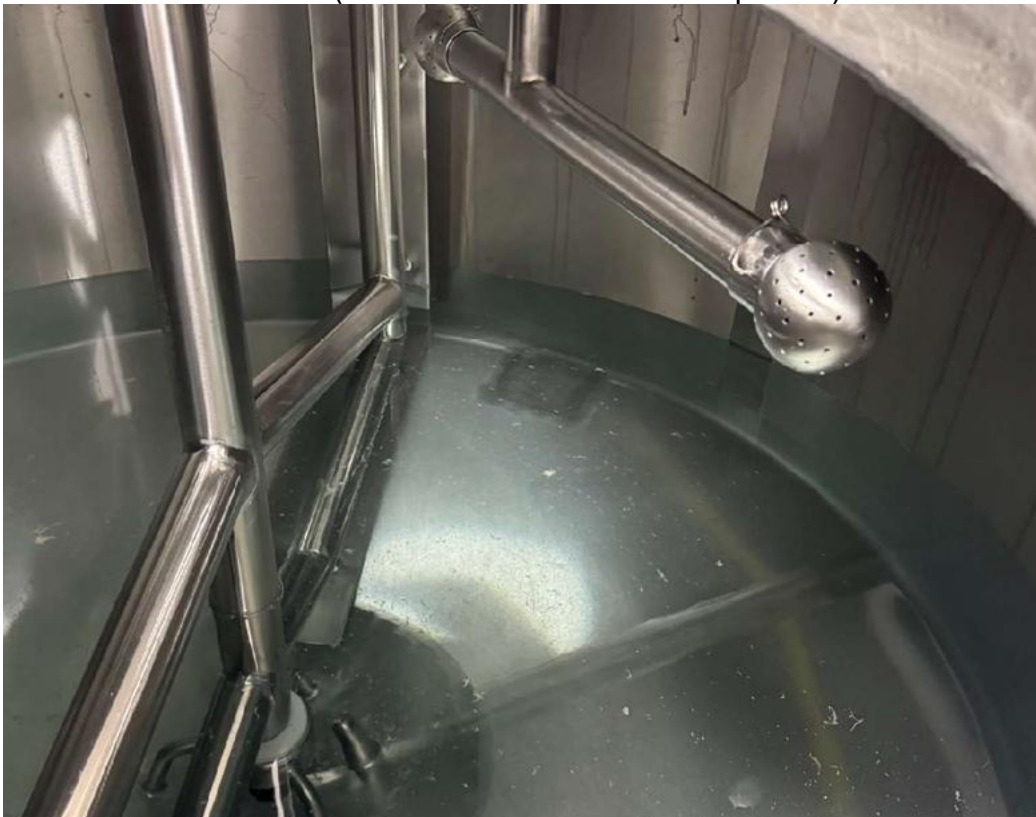
Fill level in the tank
